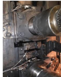
Rear view of rollers
